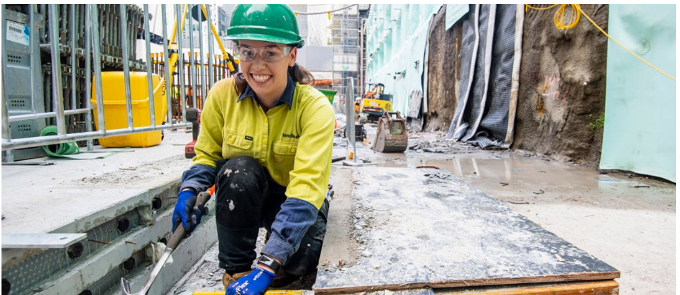
Allyssa is a formwork apprentice at the Sydney Metro Victoria Cross Station site
